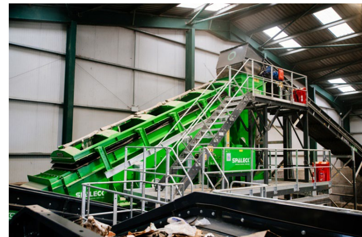
TRS Plant in the U.K.
